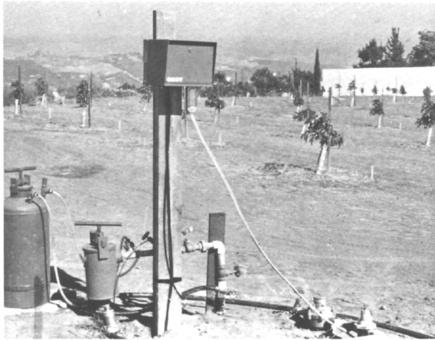
Control Center — automatic timer, fertilizer tank, screen filter, pressure gauges, \frac{3}{4} " water meter and pressure reducing valve.
