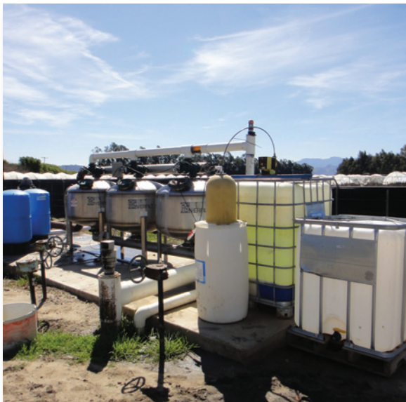
Figure 8. Filtration system on supply line improves back flush rates, and reduces water and electricity requirements.
