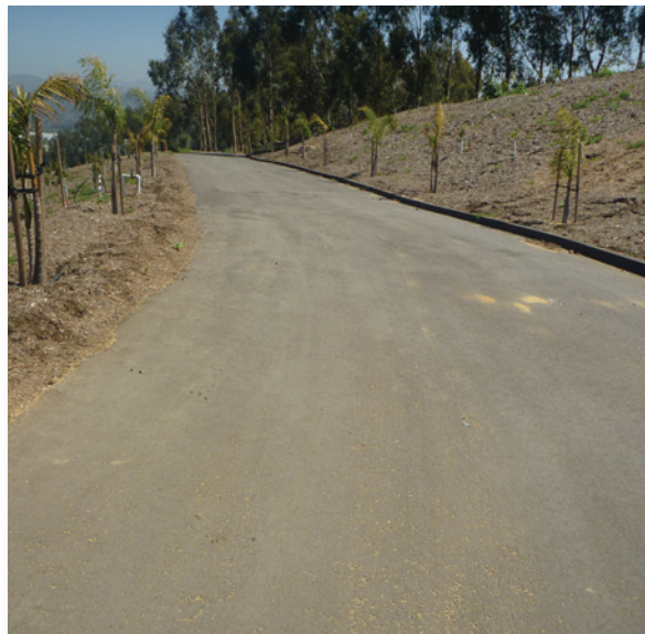
Figure 10. Paved roads eliminate dust generated by vehicular traffic and provides a protective conduit for runoff (note camber inside road with asphalt curb). Since the runoff is not flowing through a bare ditch, there will be no erosion.
