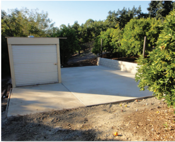
Figure 12. Concrete Pad for Equipment provides a maintenance/storage area for tractors and farm equipment. This benefits the watershed as it provides a containment area reducing the potential for engine leaks and spill from percolating into the soil.
