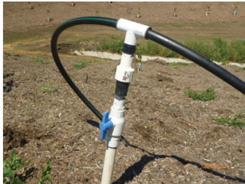
Figure 3. Pressure regulator and shut-off valve on a drip system provides water delivery to each irrigation line, despite changes in elevation. Shut-off valves at each line provide additional control to water usage throughout the orchard.
